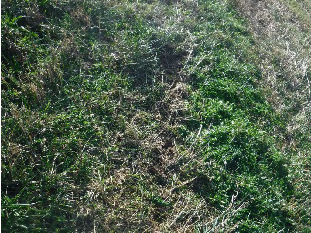
13 – Erosion Downstream Slope
