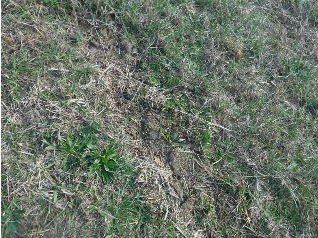
3 – Erosion Downstream Slope
