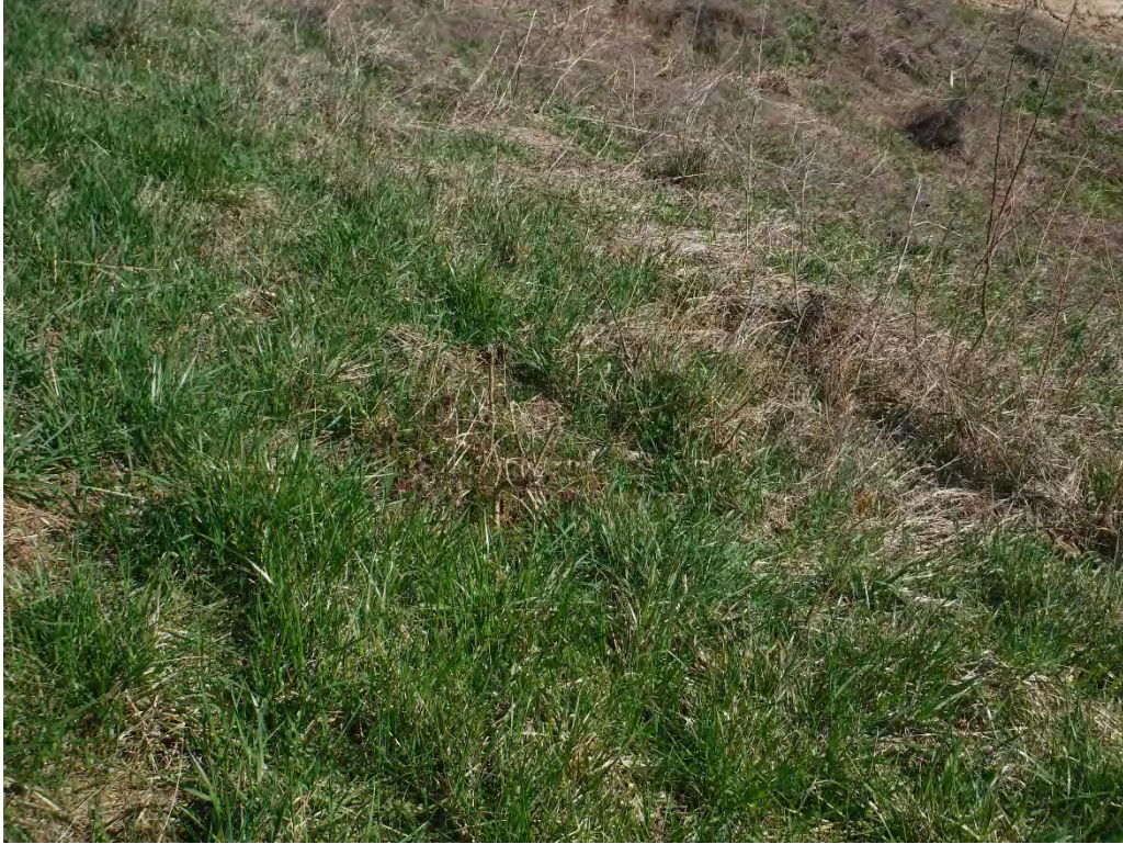
3 – Erosion Downstream Slope
