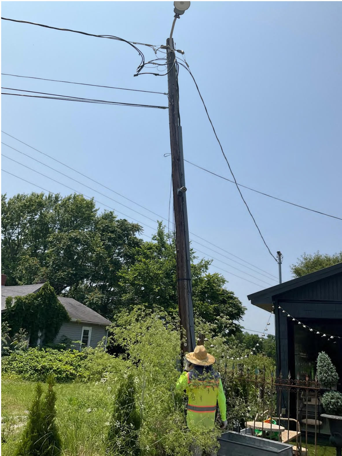
Figure 5-2: Communications attachments are above the top of the electric service riser in the power space.
