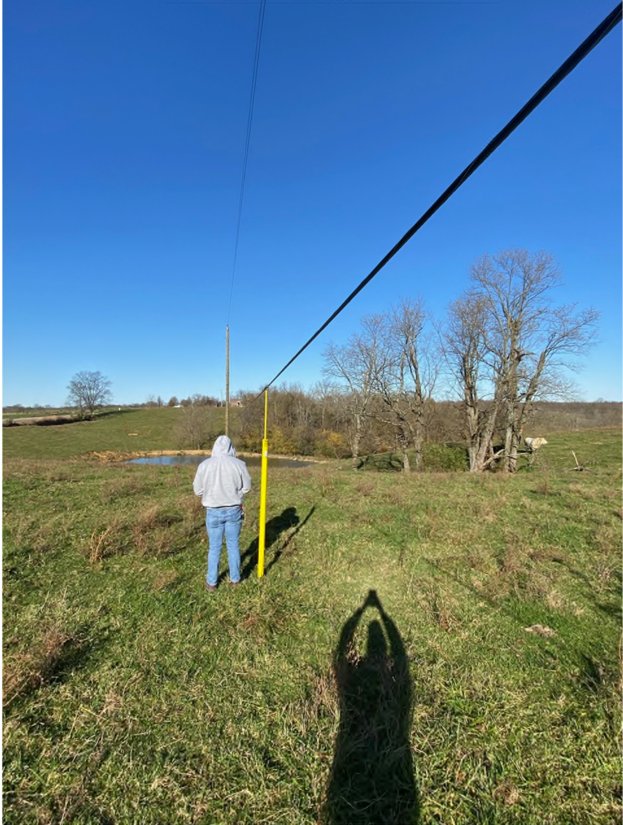
Figure 6 – Communications attachment appears to not be pulled to proper tension causing low midspan height.
